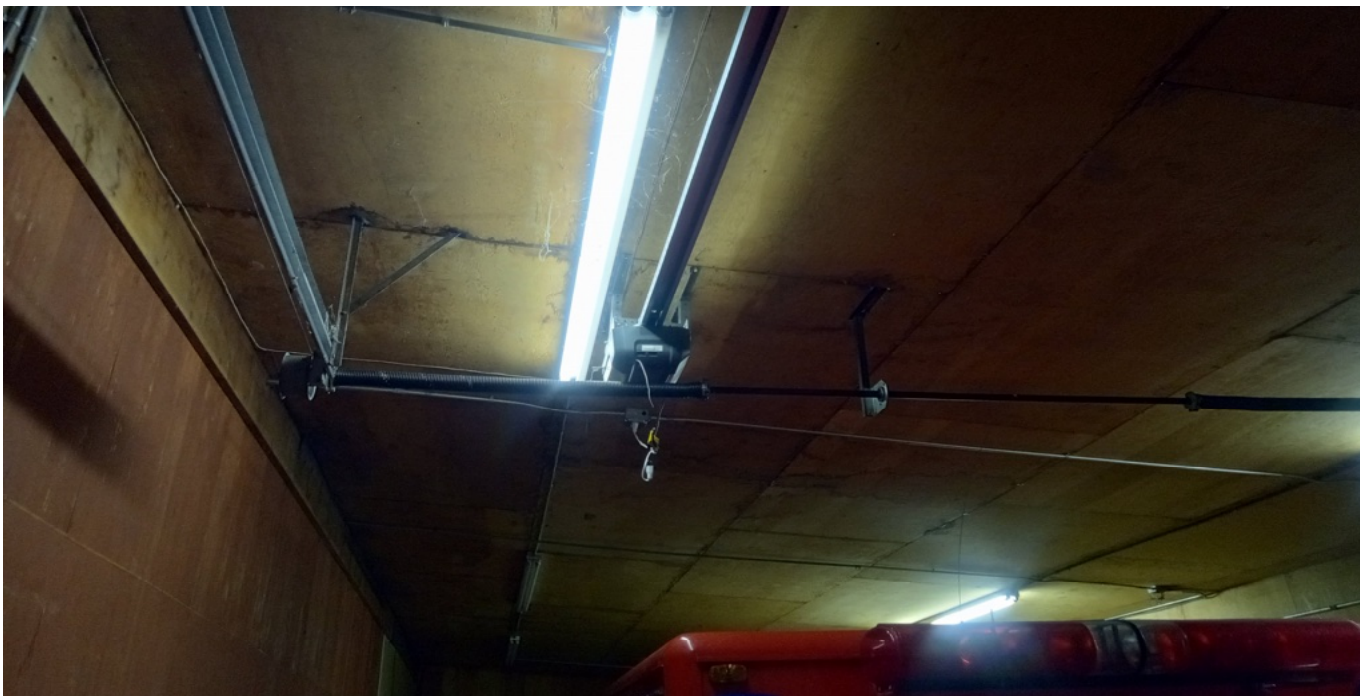
Figure 6: INADEQUATELY BRACED DOOR TRACK
